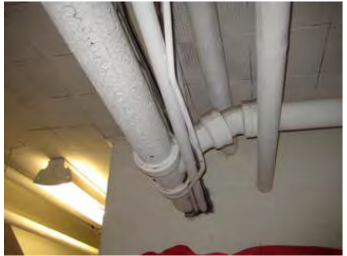
Sanitary Waste Piping
