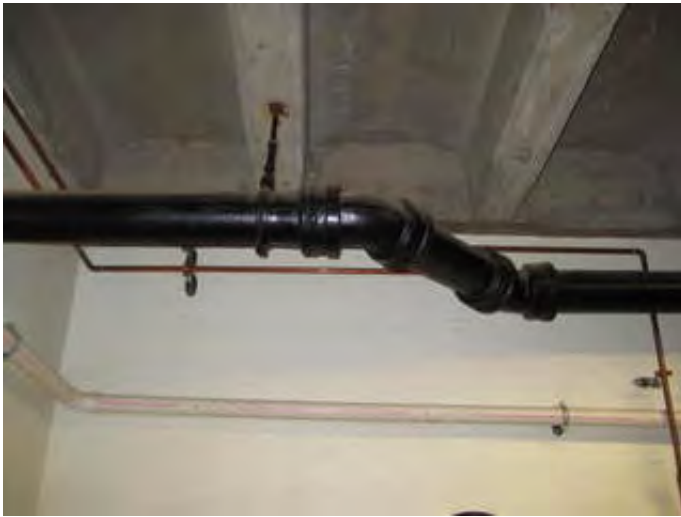
Sanitary Waste Piping
