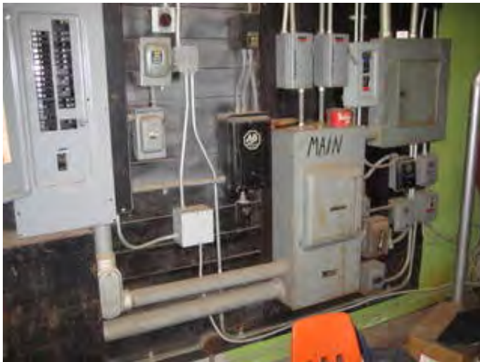
Main Electrical Distribution Panel
