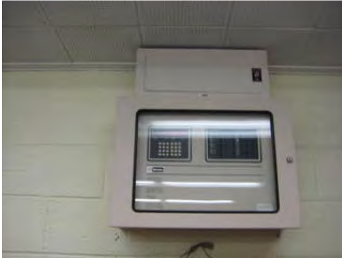
Centralized Clock System
