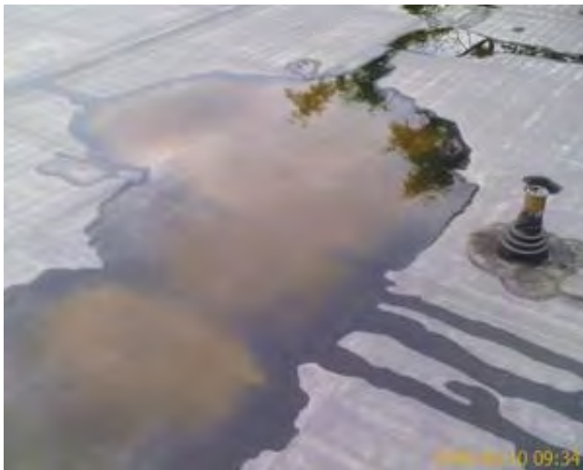
Typical Standing Water Condition
