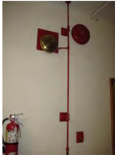
Fire Alarm Bell and Manual Pull Station
