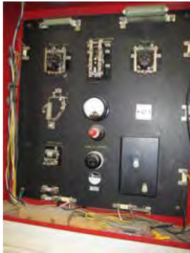
Fire Alarm Control Panel
