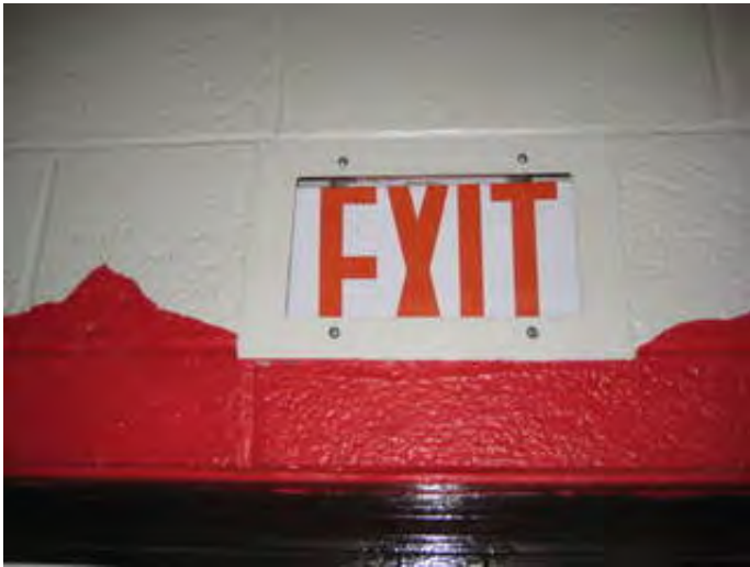
Non-Compliant Non-Illuminated Exit Sign
