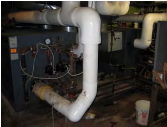
Natural Gas Fired Steam Boilers
