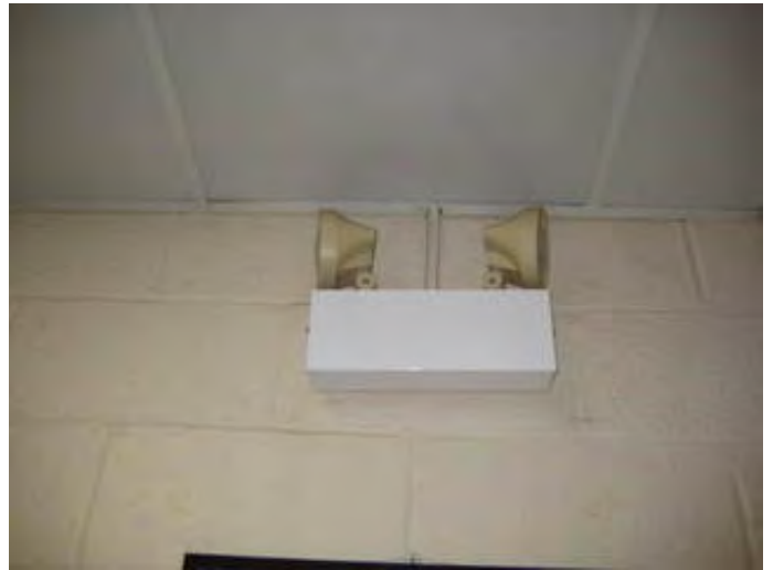
Emergency Egress Light Fixture
