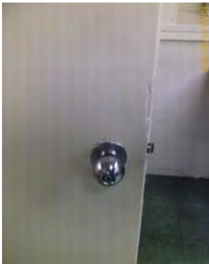
Typical Door Hardware
