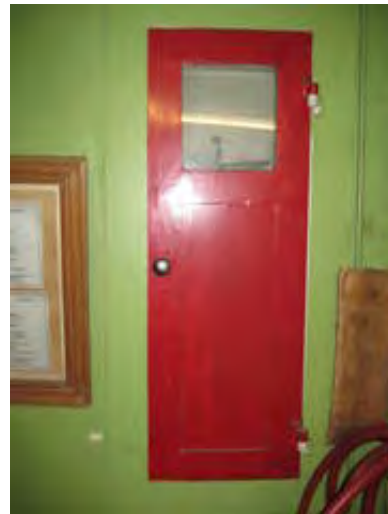
Fire Extinguisher Cabinet
