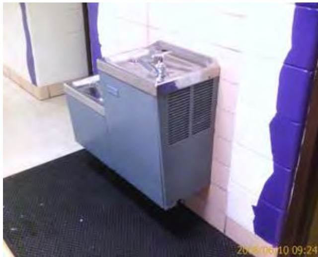
Typical Electric Water Cooler to be Replaced
