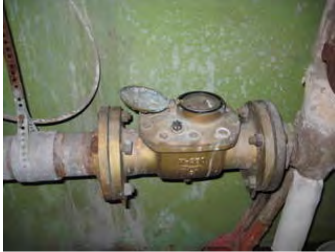
Incoming Domestic Water Meter
