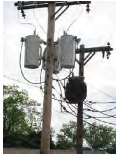
Pole Mounted Transformers
