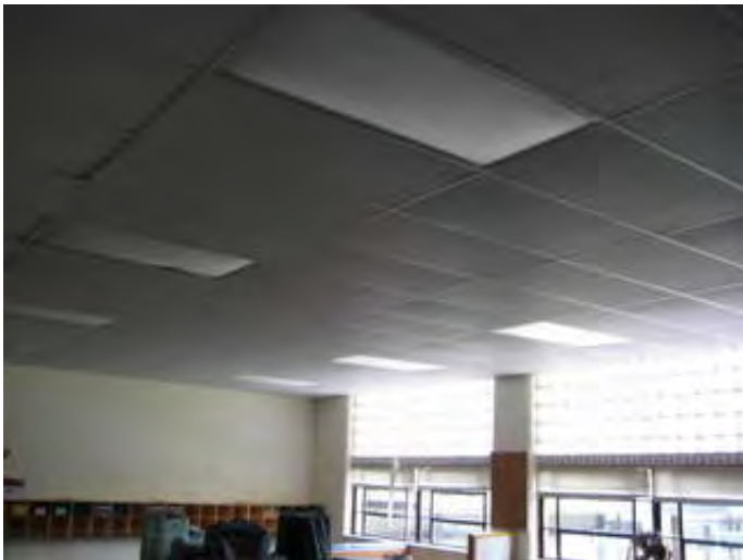
1948 Original Construction Classroom Fluorescent Light Fixtures
