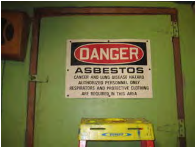
Pipe Insulation and Fittings
