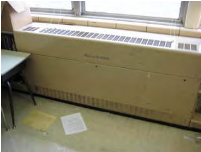
1954 Addition Unit Ventilator
