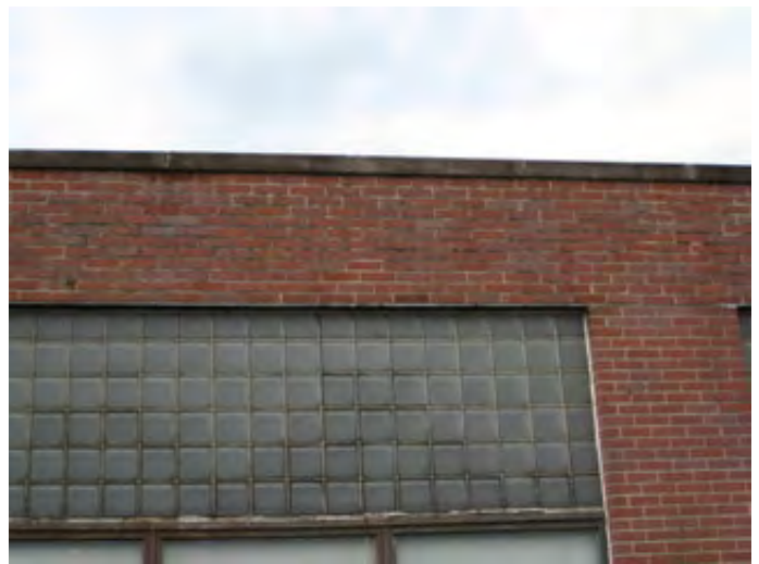
Brick Veneer Condition
