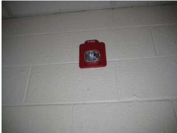
Fire Alarm Horn and Strobe Indicating Device
