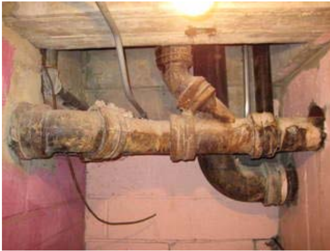
Sanitary Waste Piping
