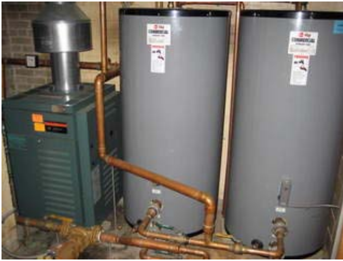
1923 Original Construction Domestic Hot Water Heater and Storage Tanks
