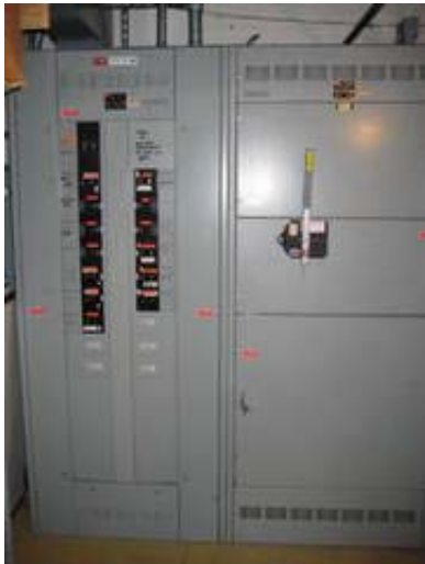
Main Electrical Distribution Panel
