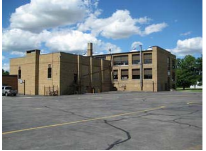
Asphalt Pavement Condition
