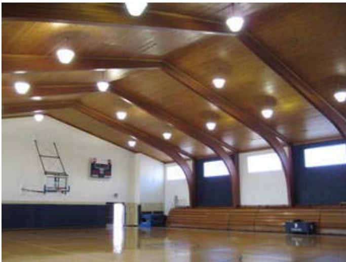
Gymnasium Metal Halide Light Fixtures
