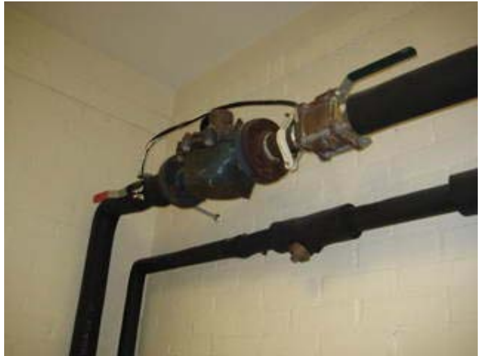
1923 Original Construction Incoming Domestic Water Service
