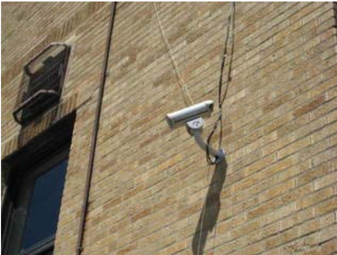
Security System CCTV Camera
