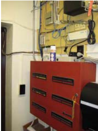
Fire Alarm Control Panel
