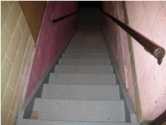
Non-Compliant Stairway and Railing
