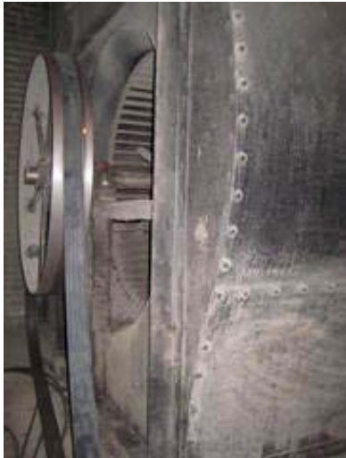
1923 Original Construction Air Handler / Central Relief Fan
