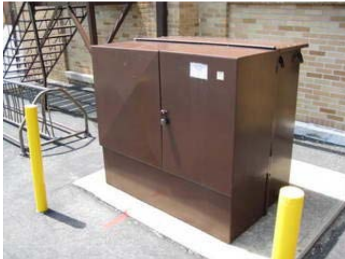
Pad Mounted Transformer
