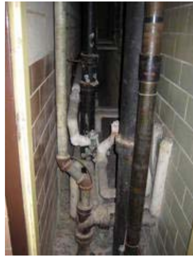
Sanitary Waste Piping
