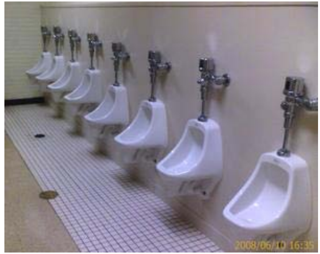
Typical Plumbing Fixture Condition
