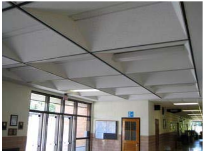
Student Dining Fluorescent Light Fixtures
