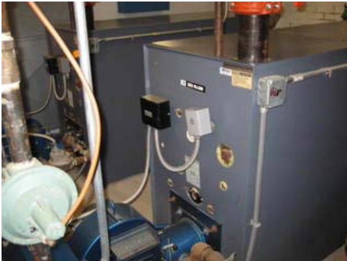
1923 Original Construction Hot Water Boilers
