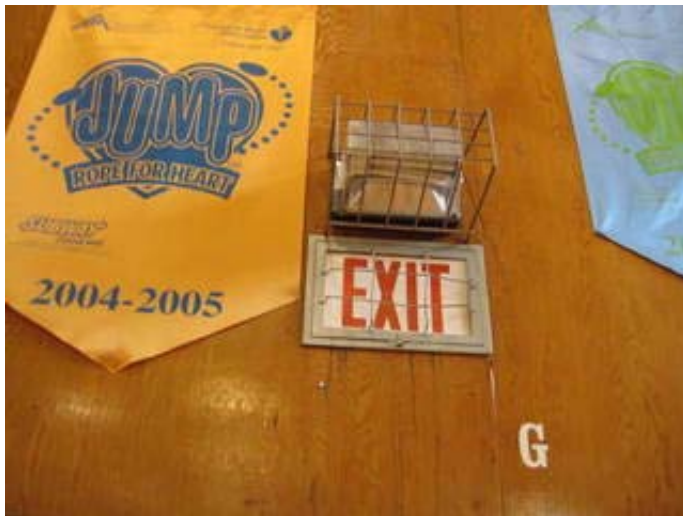
Non-Compliant Non-Illuminated Exit Sign
