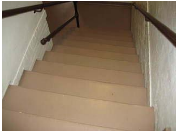
Non-Compliant Stairway and Railing
