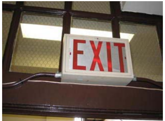
Non-Compliant Lighted Exit Sign
