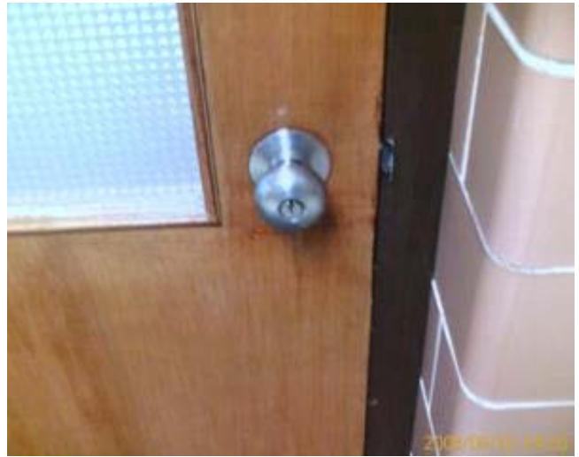
Typical Door Hardware
