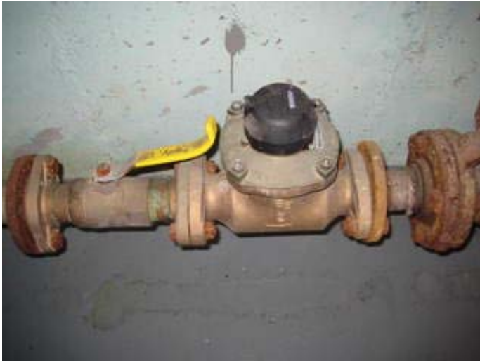
1954 Addition Incoming Domestic Water Meter
