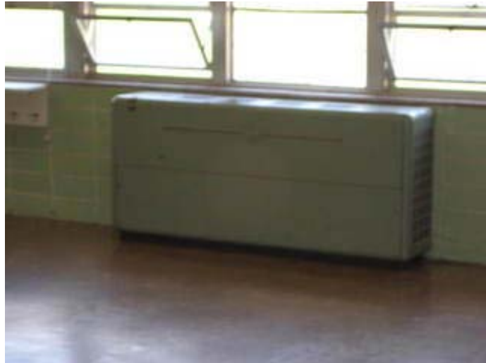
1954 Addition Steam Unit Ventilator
