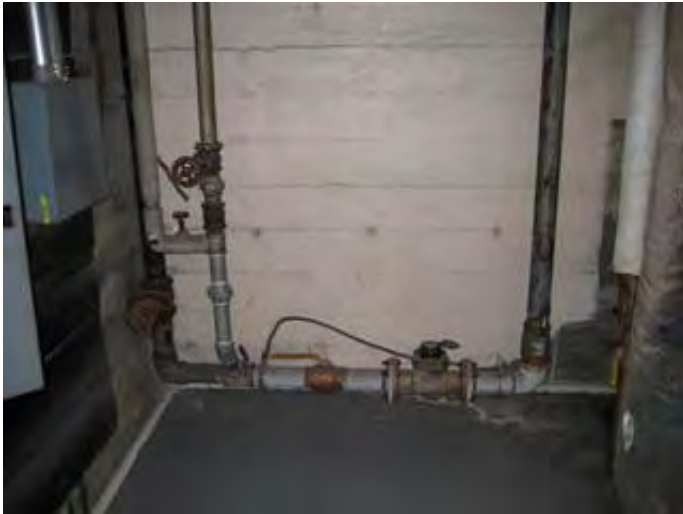
Incoming Domestic Water Service
