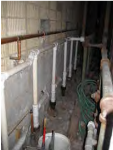
Sanitary Waste Piping
