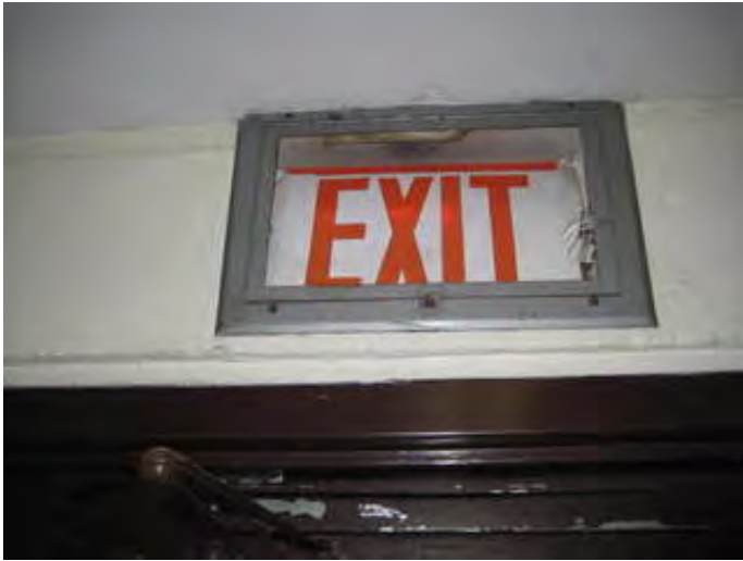
Non-Compliant Non-Illuminated Exit Sign
