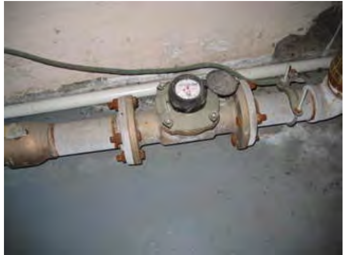
Incoming Domestic Water Meter
