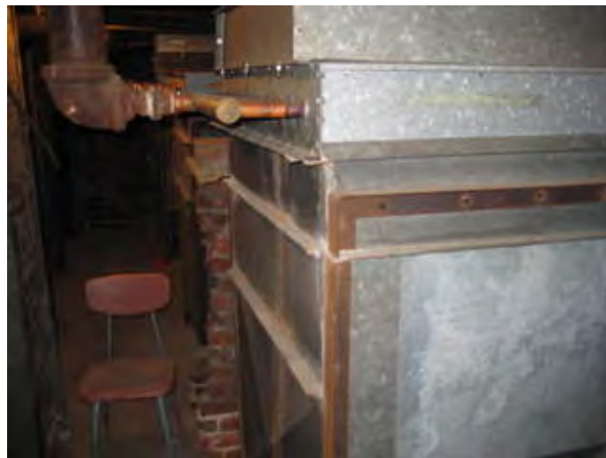
1922 Original Construction Air Handler
