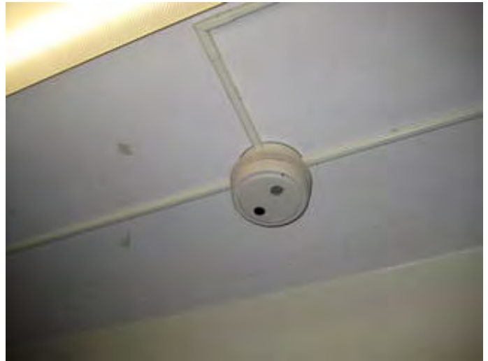
Fire Alarm System Smoke Detection Device
