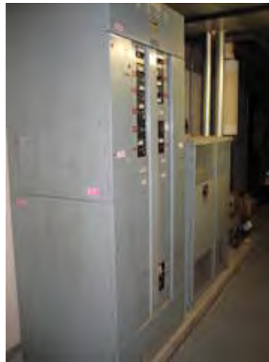
Main Electrical Distribution Panel
