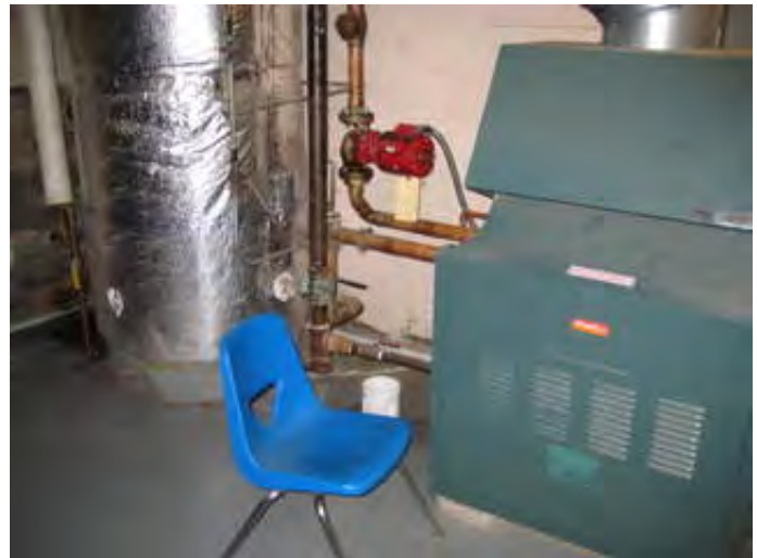
Domestic Hot Water Heater and Storage Tank
