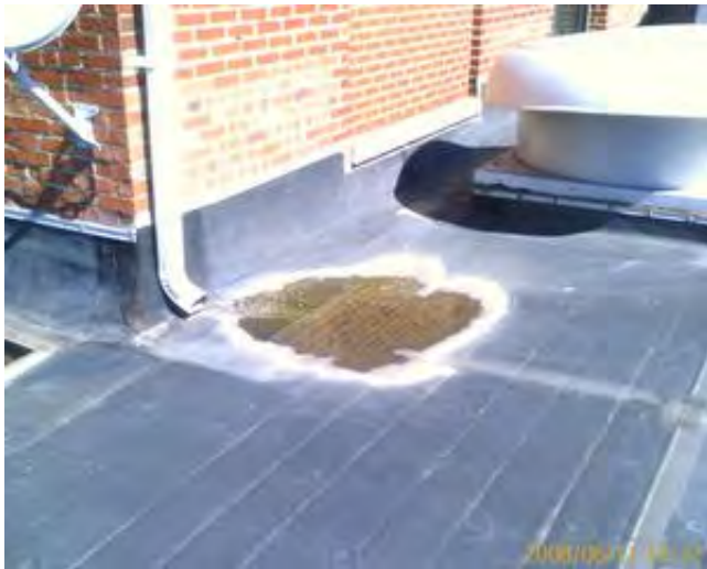
Typical Standing Water Condition
