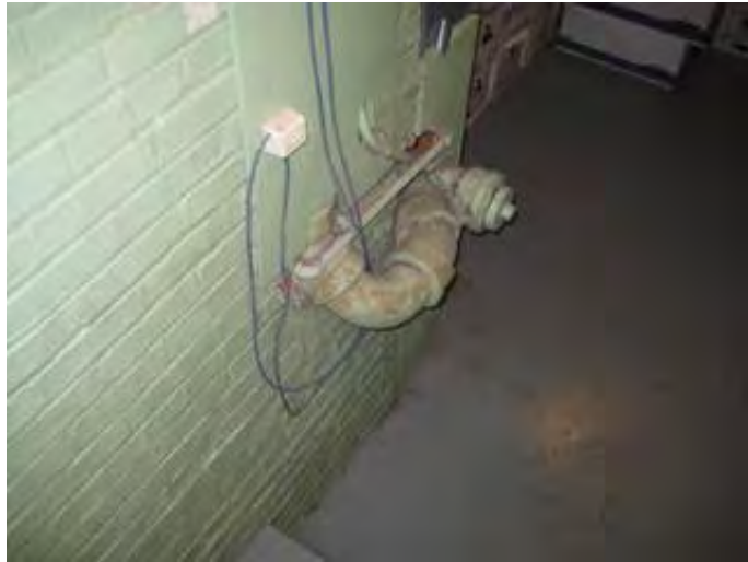
Sanitary Waste Piping
