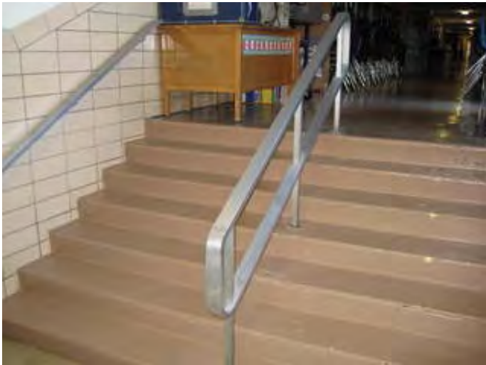
Non-Compliant Stairway and Railing
