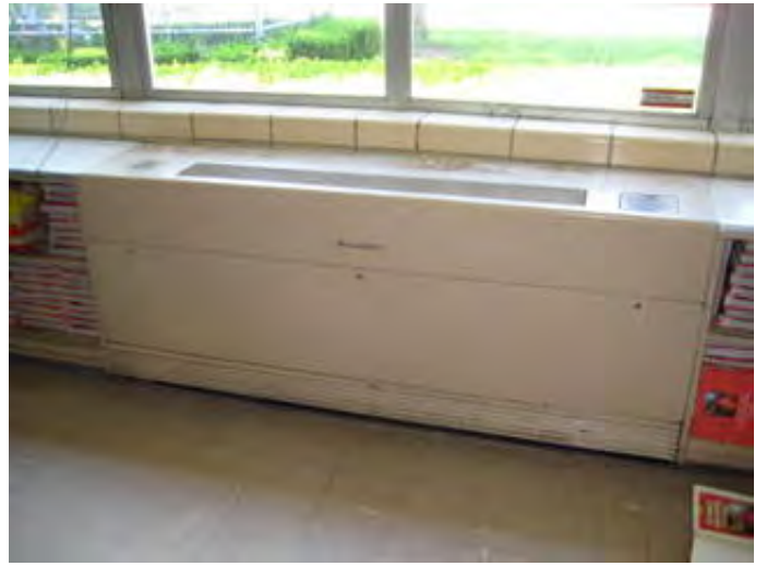
1962 Addition Steam Unit Ventilator
