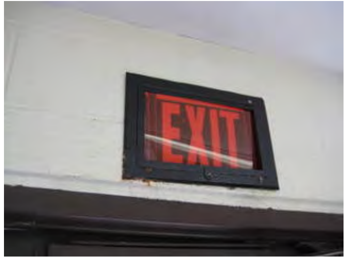
Non-Compliant Exit Sign
