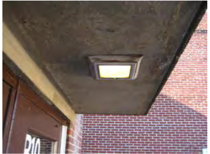
Recessed Entry Light Fixture
