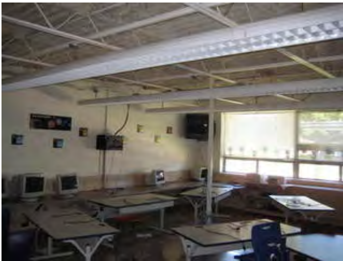
1962 Addition Classroom Fluorescent Light Fixtures
