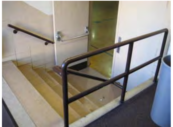
Non-Compliant Stairway and Railing
