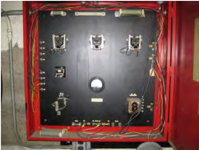
Fire Alarm System Control Panel
