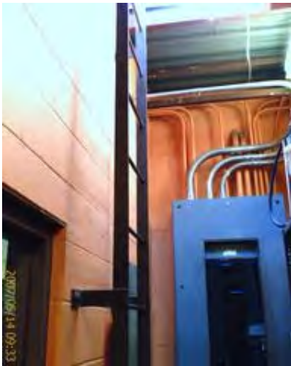
Typical Access Ladder
