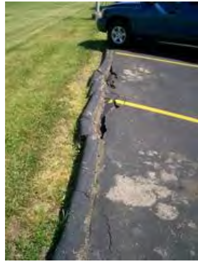
Asphalt Curb in Poor Condition
