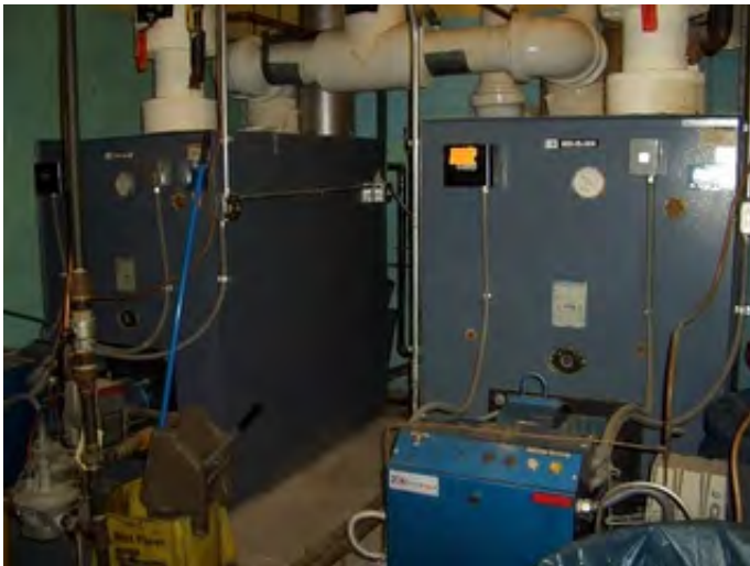
Heating Water Boilers
