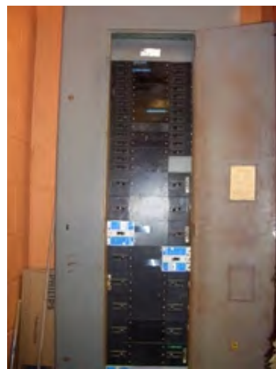
Electrical Sub Panel
