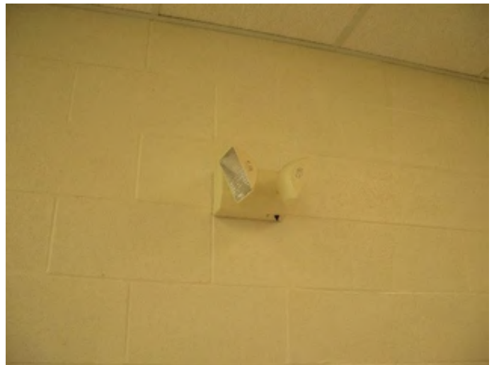
Emergency Light Fixture
