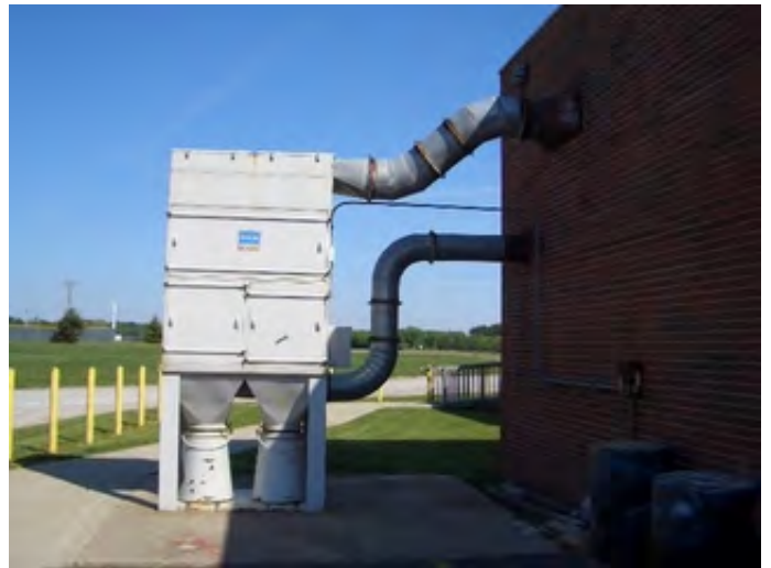
Dust Collection System
