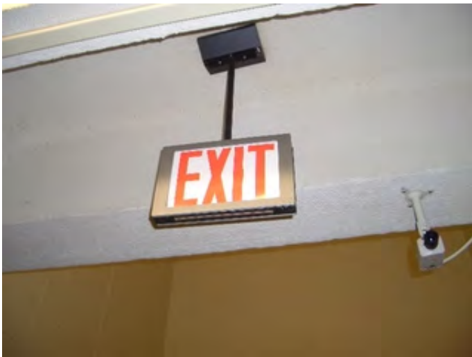
Lighted Exit Sign
