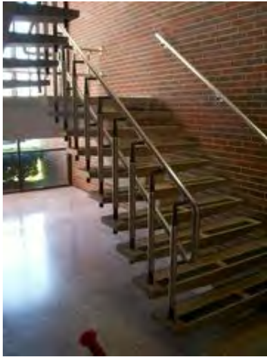
Non Compliant Stair Towers and Railings
