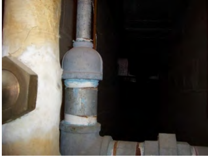
Galvanized Water Piping
