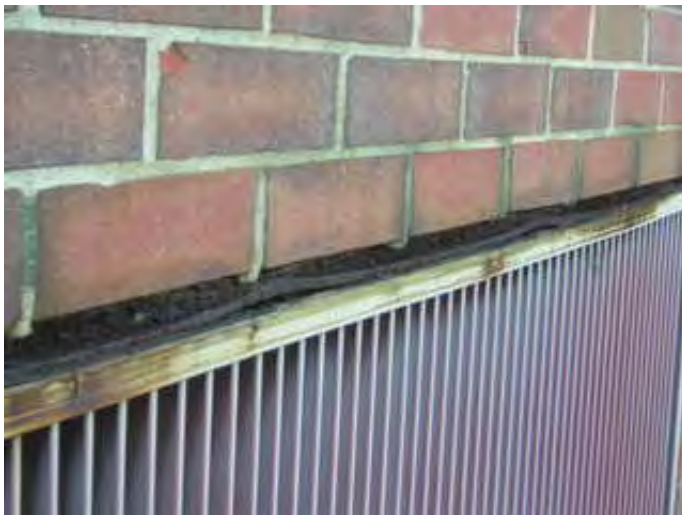
Deteriorated Lintel Above Wall Grille
