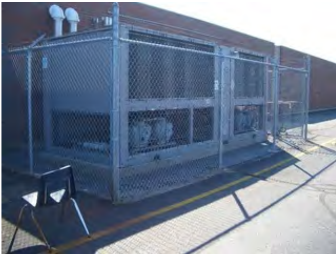
Air Cooled Chiller
