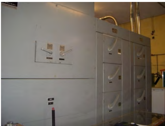
Main Distribution Panel
