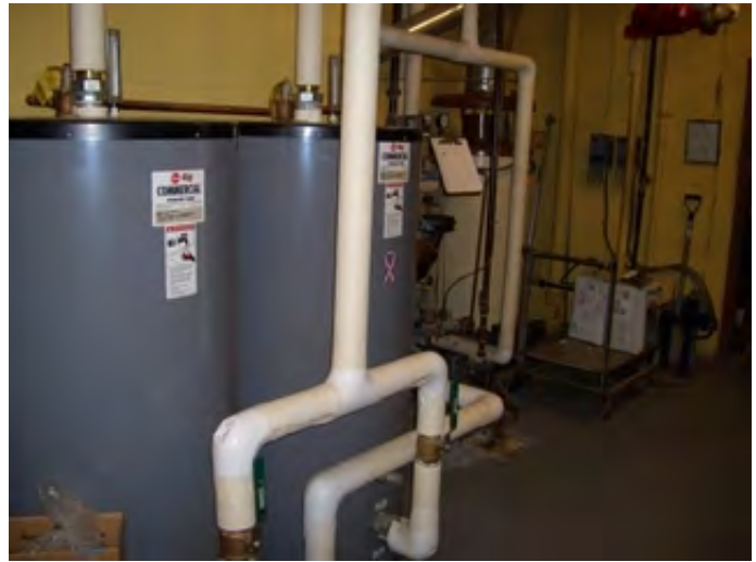
Domestic Water Heating System
