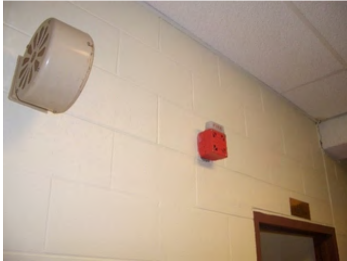
Fire Alarm Horn and Strobe Device
