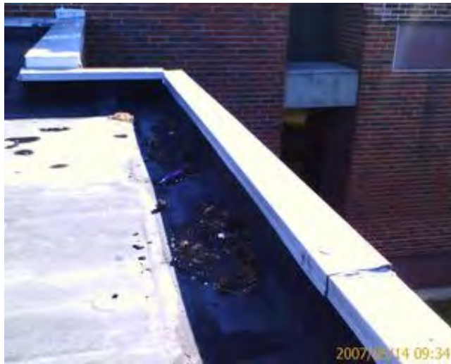
Typical Coping Condition
