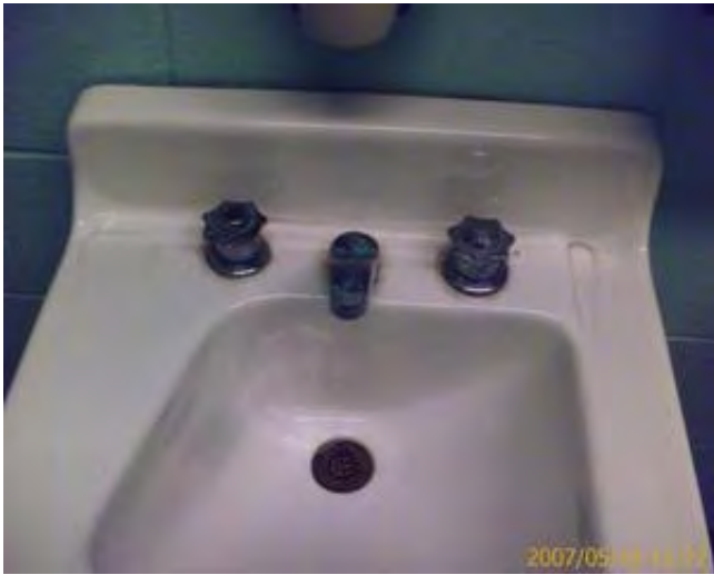
Typical Lavatory Faucet Condition
