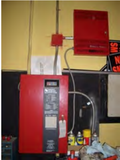
Fire Alarm Control Panel
