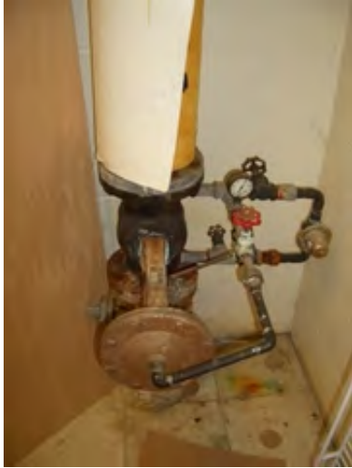
Incoming Water Main
