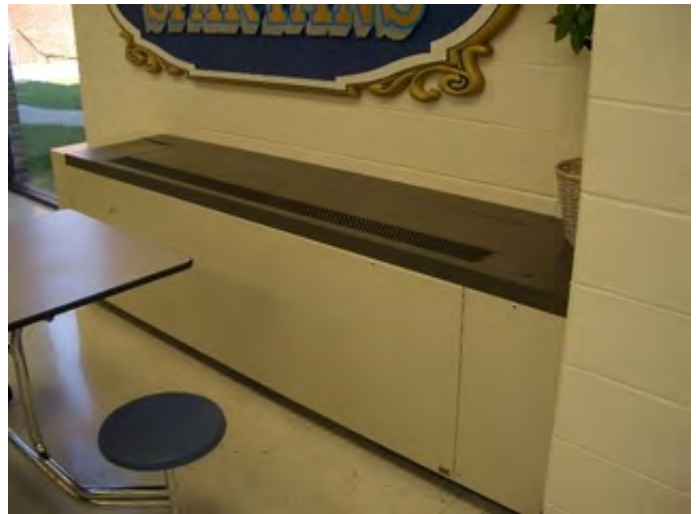
Unit Ventilator in the 2000 Addition
